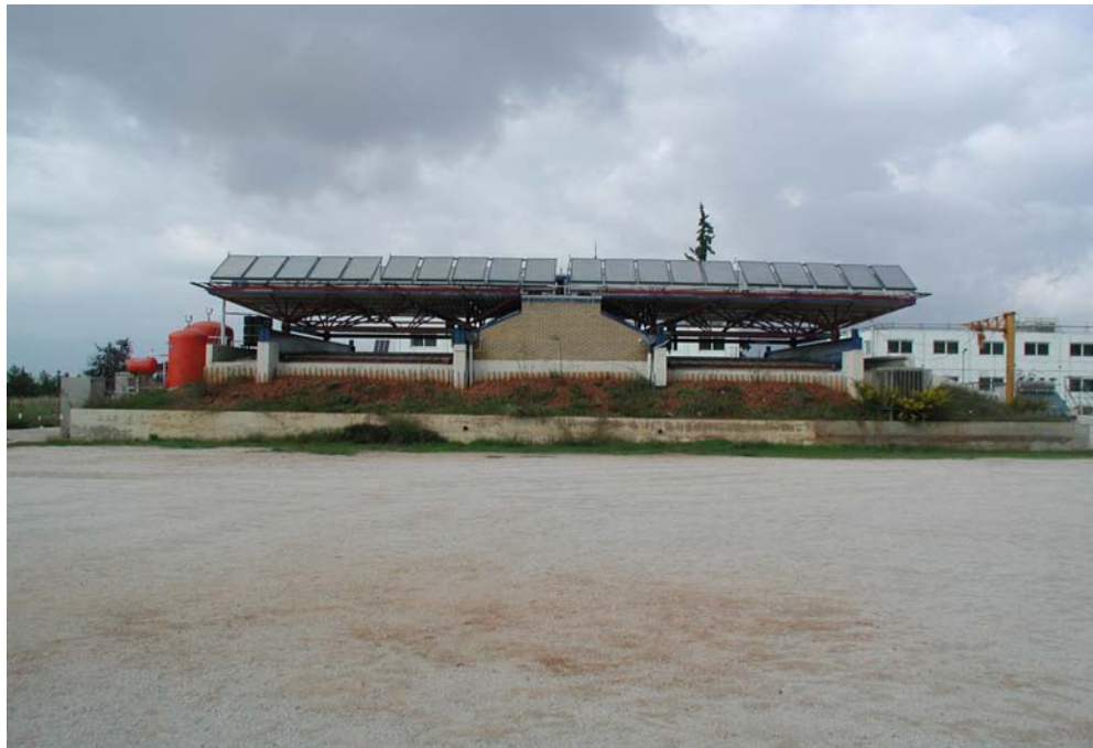
Figure 1: Panoramic view of the solar collector field as installed on the building roof
