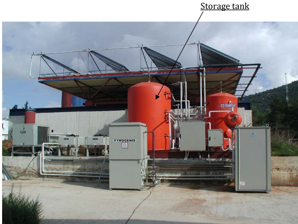
Figure 6: Lateral view of the solar collector field with the storage tank and the electrical and control panel boards
