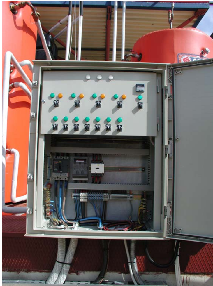
Figure 14: View of the main control panel
