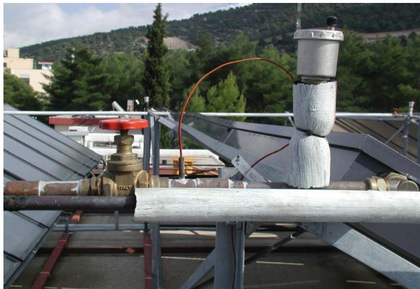
Figure 11: Detailed view of the collector outlet flow pipe showing the automatic venting valve, the thermocouple temperature sensor and the shut-off valve assembly.
