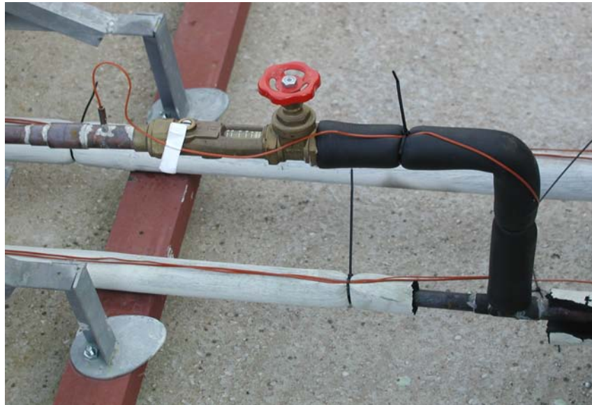
Figure 10: Detailed view of the collector inlet flow pipe showing the regulation valve, the balancing valve and the thermocouple temperature sensor assembly.
