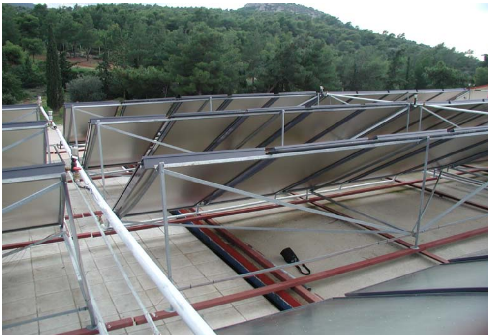
Figure 3: View of the rear side of the solar collector field
