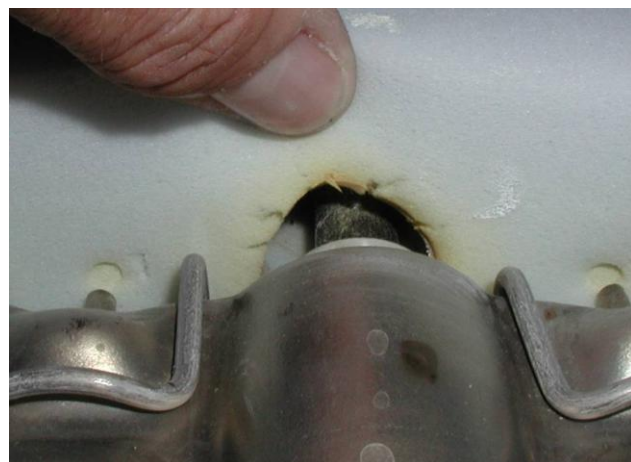
Picture 32) Insulation at the heatpipe in manifold casing
