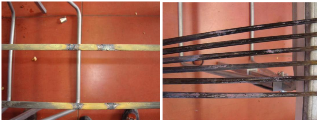
Figure 7,8 : Corrosion observed in the copper heat pipes
