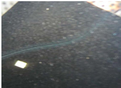
Figure 21: view of the water tear residues at the inner side of the cover
