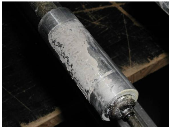
Picture 34) Dried out heat transfer paste on aluminium tube at condenser (after one year exposure before renewing paste)
