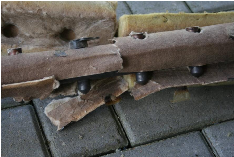
Picture 37) clam-shell insulation of manifold at final inspection
