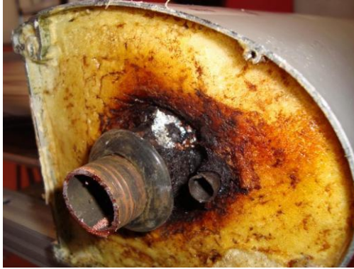
Figure 6 : Color changing and some degradation in the collector insulation
