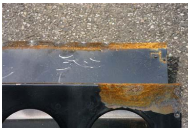
Figure 9 Corroded collector box. Manifold casing after exposure test
