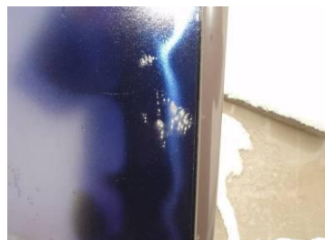
Figure 17 Cracking on absorber coating
