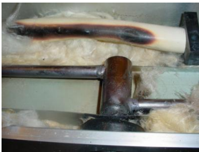
Figure 18 Deformation of absorbers tubes and headers
