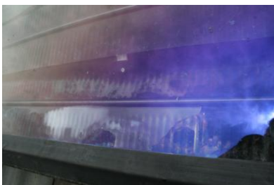
Figure 16 Cracking on absorber coating
