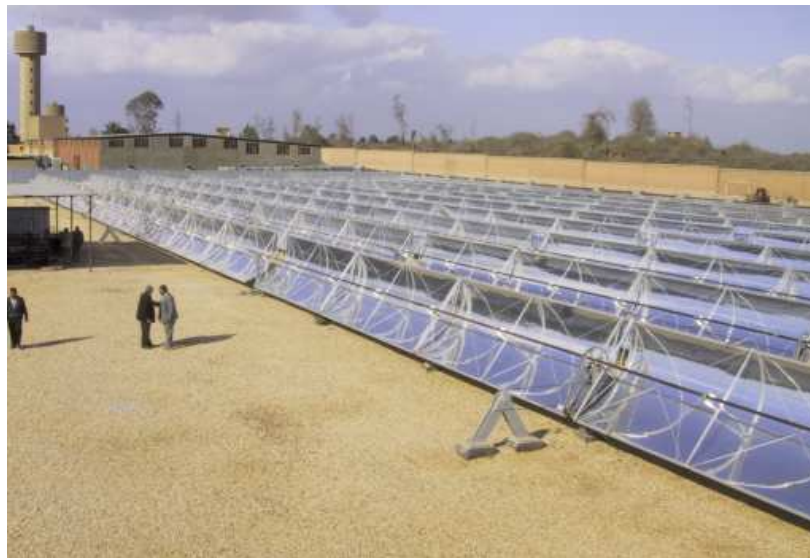
Figure 8: El NASR Pharmaceutical Chemicals, Egypt. Installed capacity: 1,33 MW th Source: Fichtner Solar GmbH. Germany
